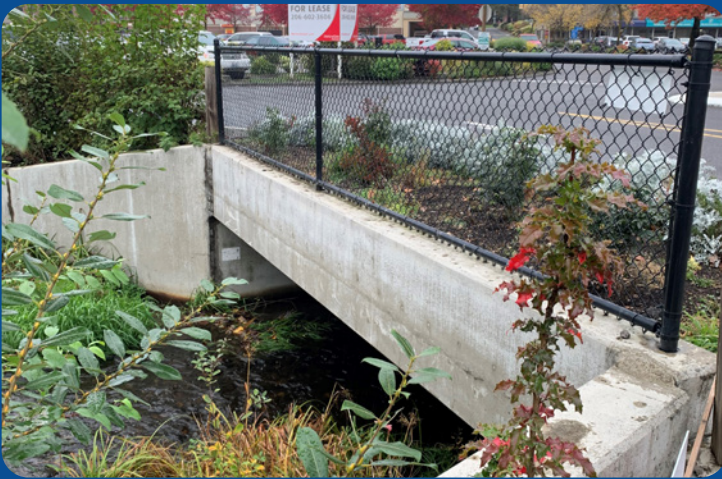
Culvert with a protective headwall that prevents erosion and allows water to pass under a road
