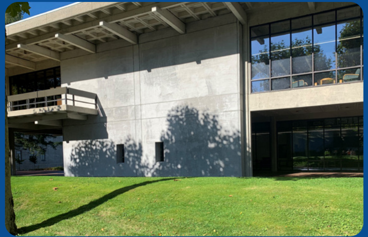
Shear wall that is part of a seismic retrofit of a university library
