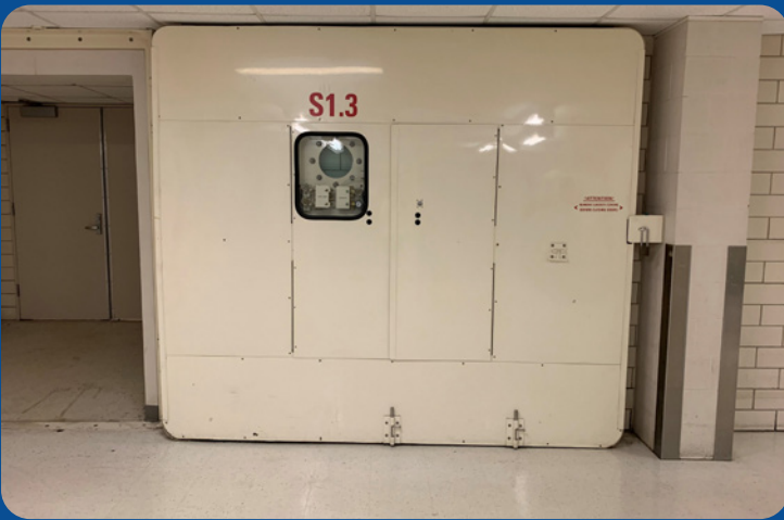
Watertight enclosure to prevent floodwater damage
